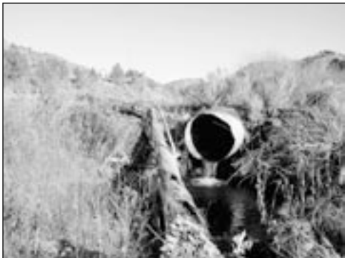
A Pine Creek culvert that was a barrier to fish, before its removal in 2002
